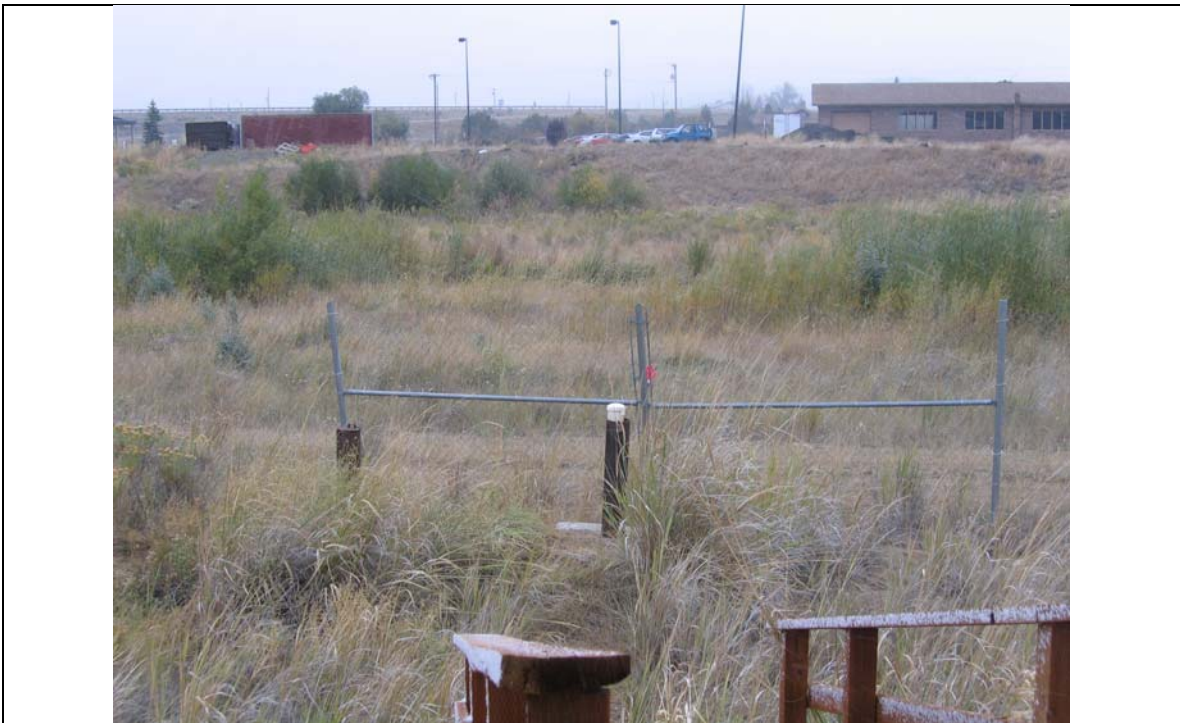
Photo 6. Damaged gate and well with frost heaving.
