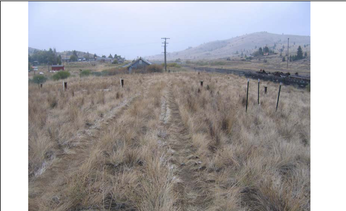
Photo 10. Tire ruts on repository cap.
