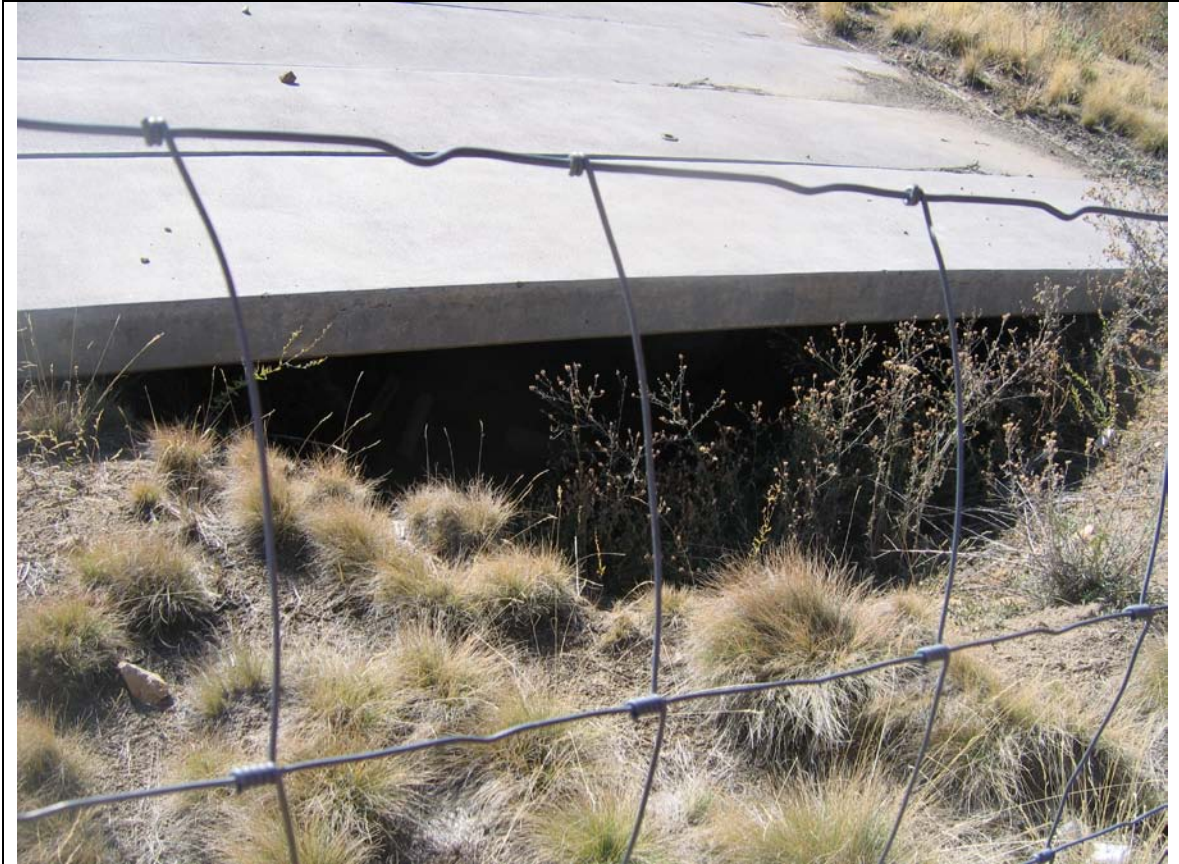
Photo 12. Otisco Shaft cover compromised. (Note that a physical hazard such as a mine shaft is not addressed under CERCLA.)
