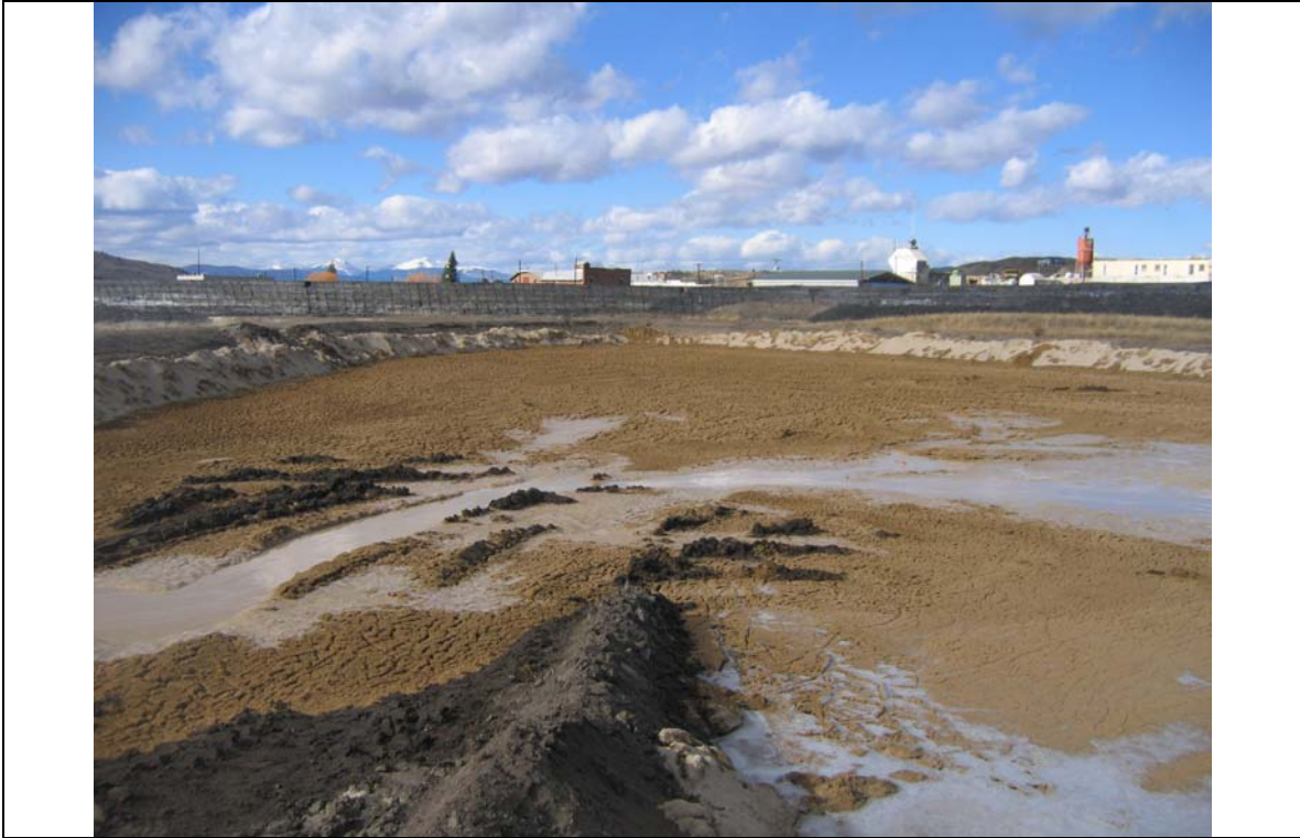
Photo 5. Sludge Drying Bed at Lower Area One
