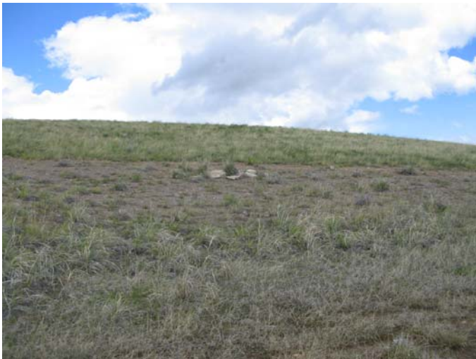
Photograph 5757. Sparsely vegetated portion of the Flue Dust repository cap. RDU 14 - Smelter Hill Facilities Area WMA.
