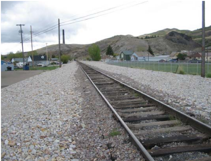
Photograph 5739. Rock cap and retaining wall in Anaconda to prevent contaminated sediment from getting onto the city street. RDU 5 – Active Railroad/Blue Lagoon. (Community Soils OU remedy)
