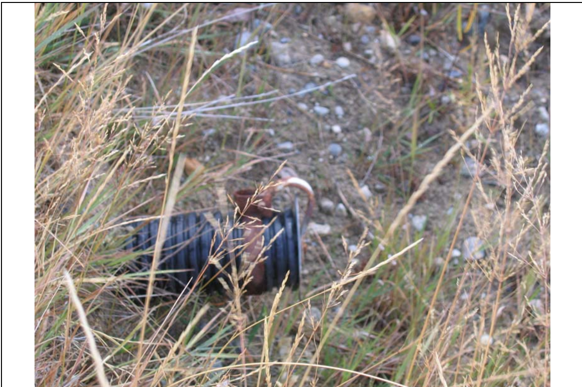
Photo 6. One of many toe drains along Pond 3 dam adjacent to Mill-Willow Bypass.
