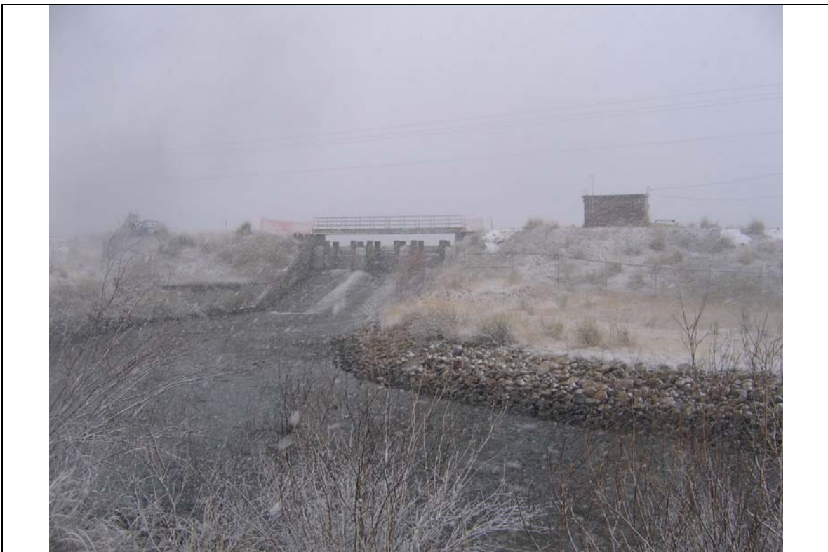
Photo 8. Pond 2 discharge hydraulic control structure (station SS-5).
