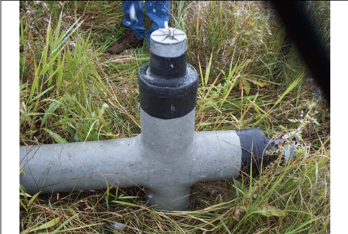
Photo 9. Manifolded Toe Drain.
