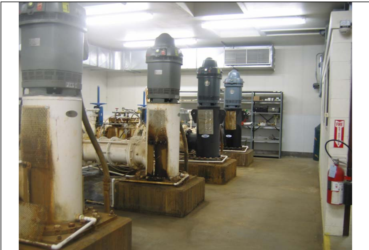
Photo 10. Groundwater interception channel pump house.
