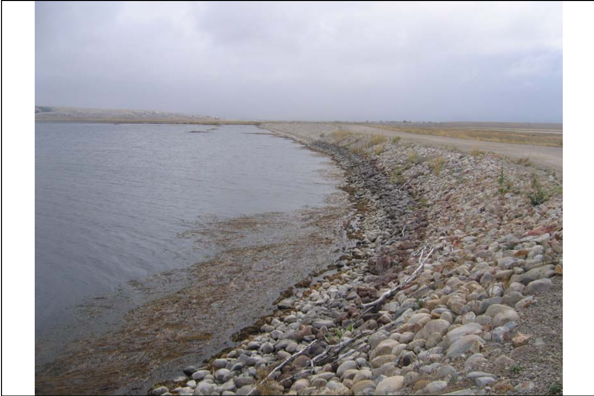
Photo 7. Riprap repair work to protect against wave run-up along banks of Pond 2.
